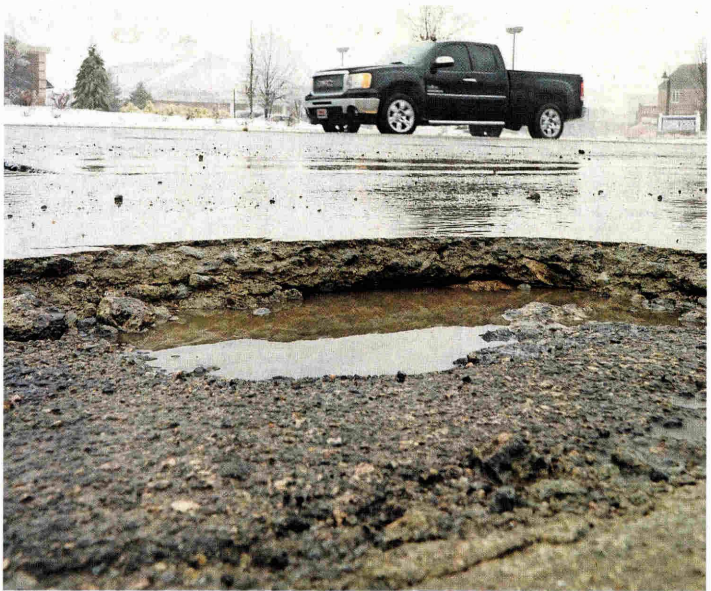
A pothole four inches deep with sharp rim lies along Canton Center Road's northbound lane. JOHN HEIDER/HOMETOWNLIFE.COM
