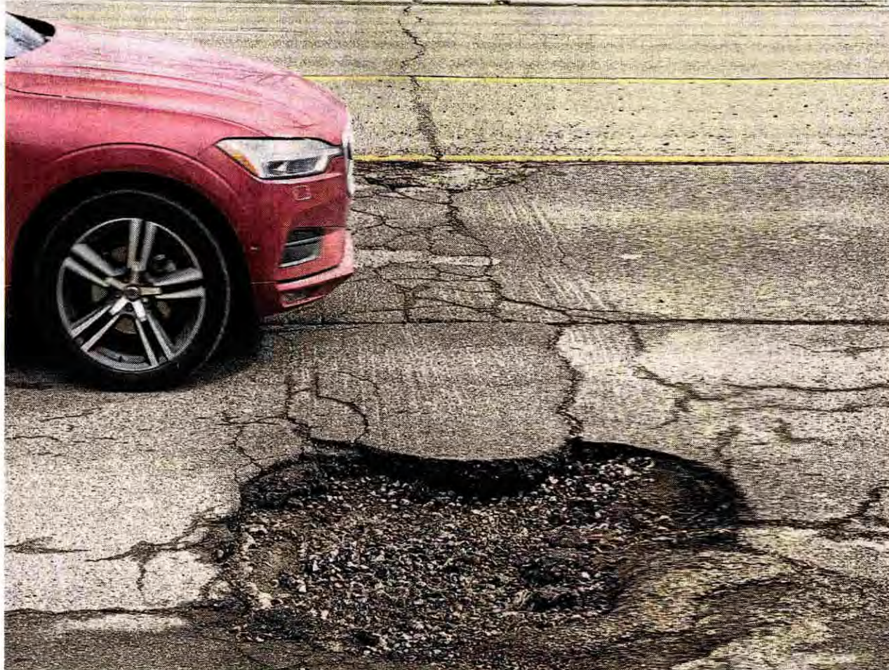
A substantial pothole in the southbound lane of Haggerty as it approaches Seven Mile. JOHN HEIDER/HOMETOWNLIFE.COM
