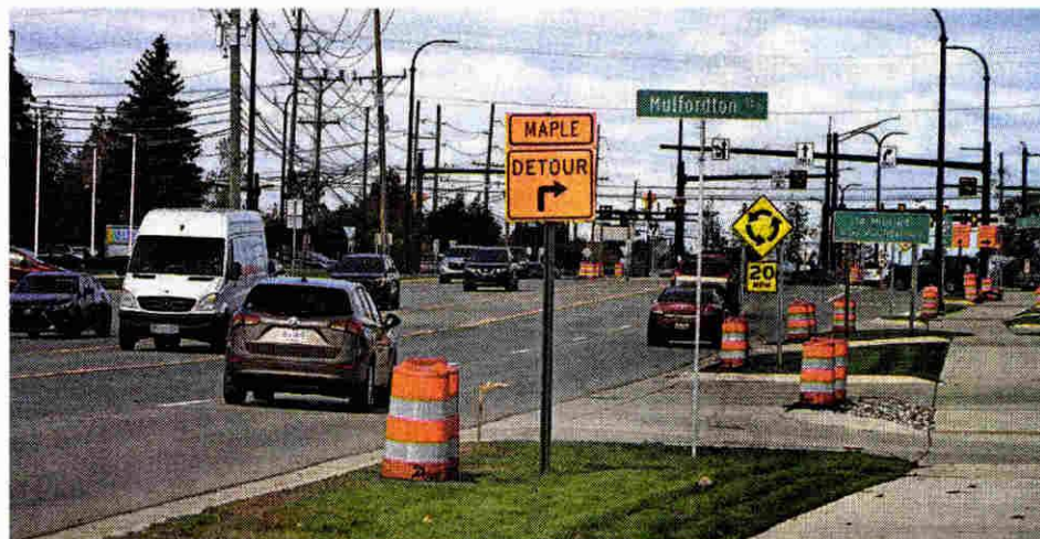
A boulevard divider lane will be constructed on this stretch Orchard Lake Road in Farmington Hills. JOHN HEIDER/HOMETOWNLIFE.COM
