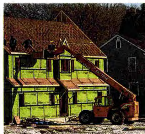
A market-rate housing development is under construction at 175 James St., a former brownfield.
