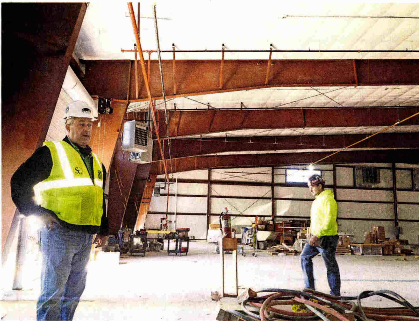
Director of Public Service for Livonia Donald Rohraff, left, stands inside the city's new DPW building May 12. The garage alone, with no support posts getting in the way of the large vehicles that will use it, takes up 21,000 square feet.
