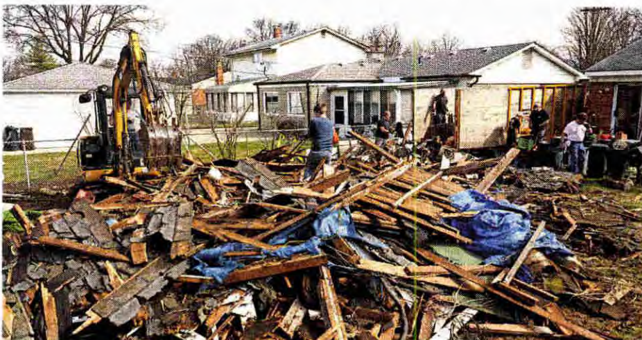
Volunteers work to sort the remains of the garage in Livonia on March 24.
