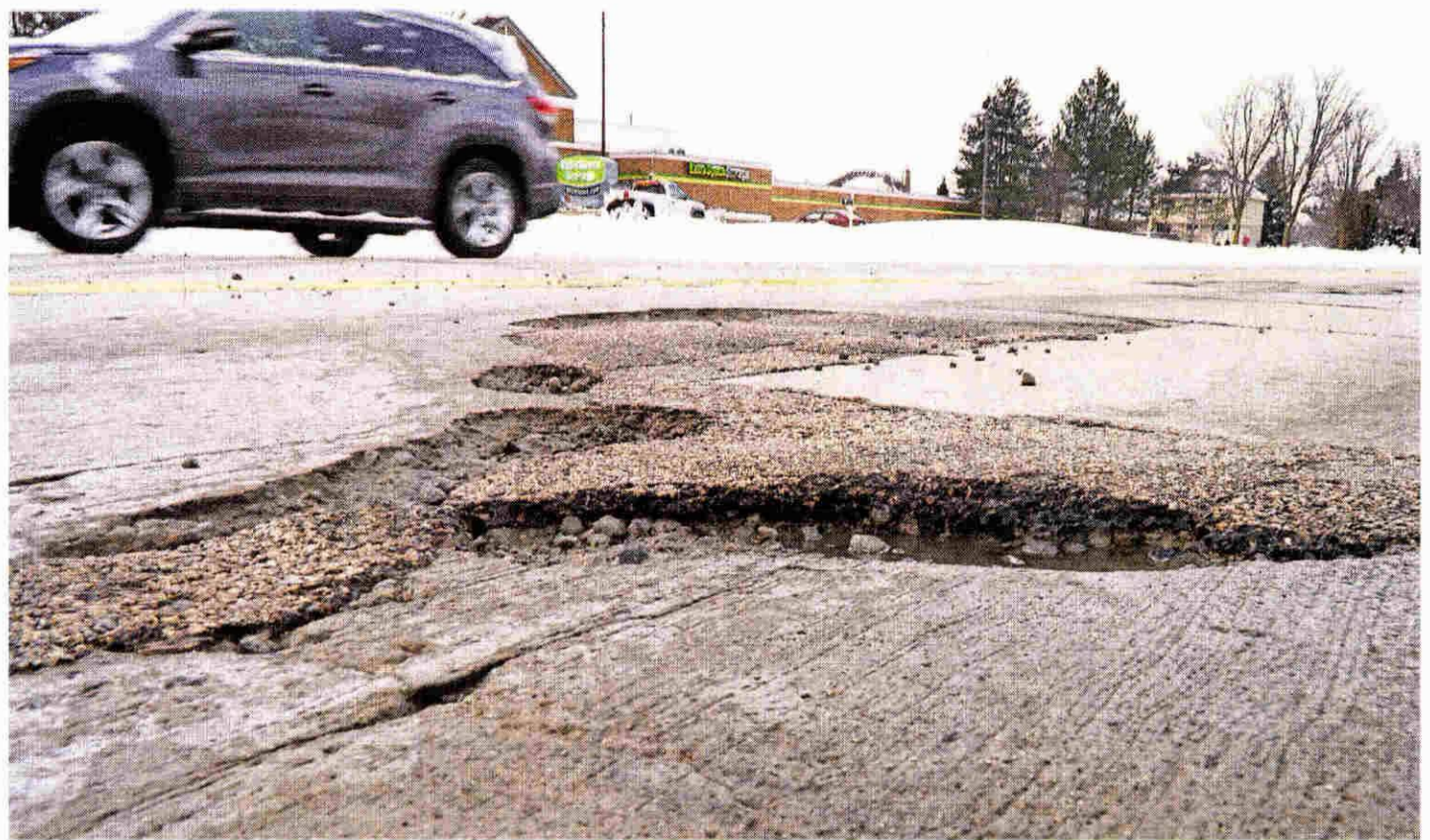
Plenty of these sharp-edged potholes await drivers along Canton Center Road near Warren. JOHN HEIDER/HOMETOWNLIFE.COM
