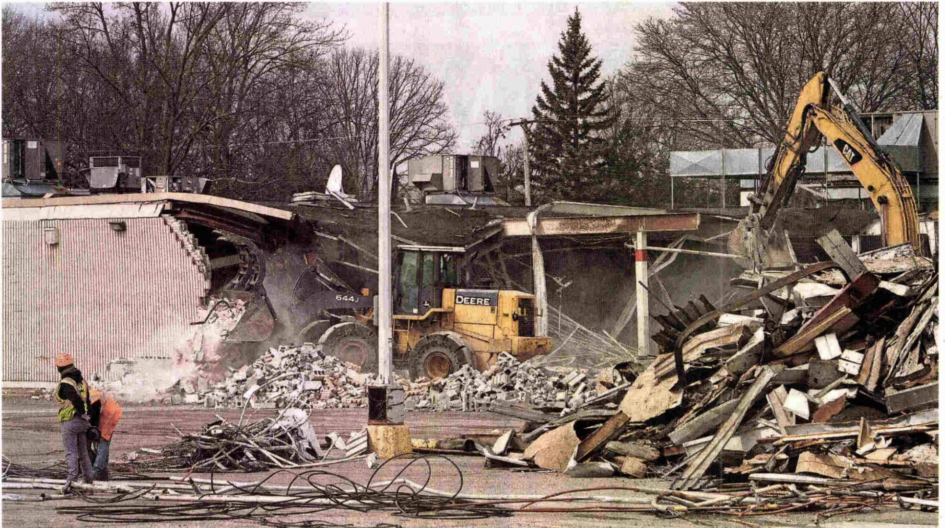
As a backhoe grabs pieces of steel beam, a bulldozer punches a dusty hole in the wall of the former Garden City Kmart. The building at Ford and Middlebelt roads, home of the first Kmart store, opened in 1962. LA Fitness bought the property and plans to build a gym there in the coming months. JOHN HEIDER/HOMETOWNLIFE.COM
