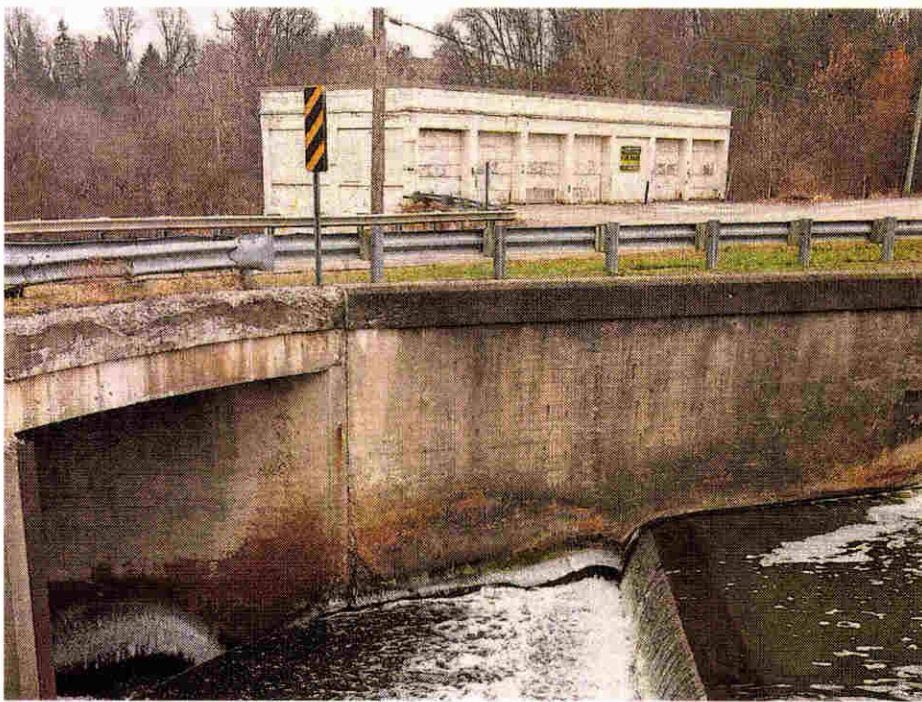
The Wilcox Mill building sits several hundred feet from the Wilcox Lake dam.
