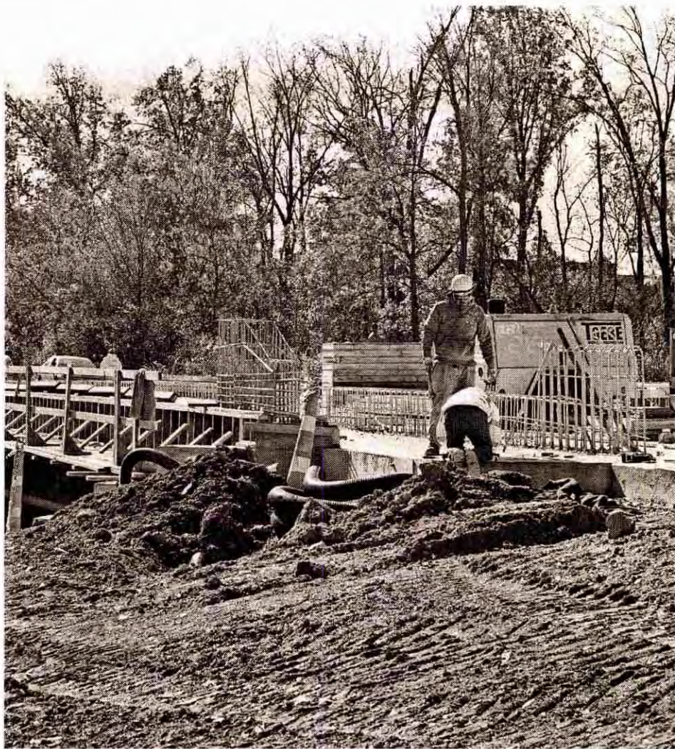
Work continues Oct. 23 on the replacement of a bridge on Lilley Road just north of Michigan Avenue in Canton Township. JOHN HEIDER/HOMETOWNLIFE.COM
