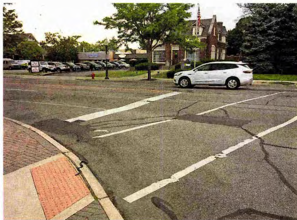
The intersection of Church and Main streets in Plymouth could use some TLC. ED WRIGHT/HOMETOWNLIFE.COM
