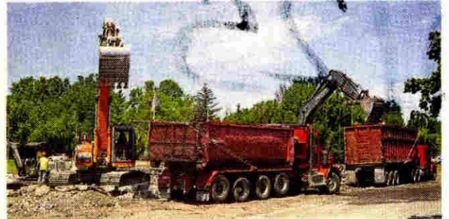
Dump trucks line up to cart debris away from the old courthouse in Farmington off 10 Mile on Aug. 14. Demolition is expected to be completed this week.
