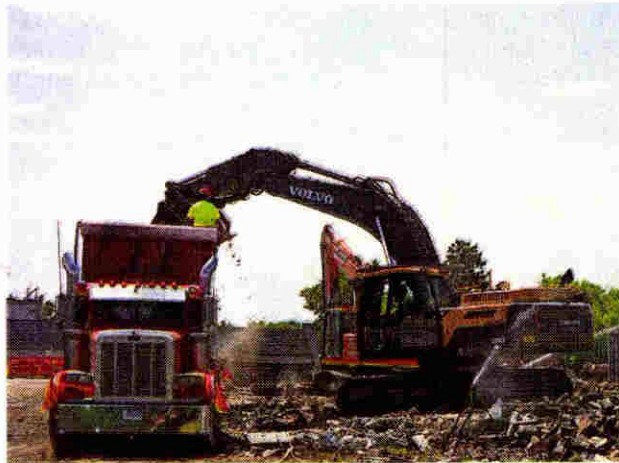
A worker supervises as debris from the old courthouse is loaded onto a dump truck for removal.
