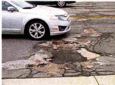
A car passes by some heavily patched pavement on Merriman in Livonia.
