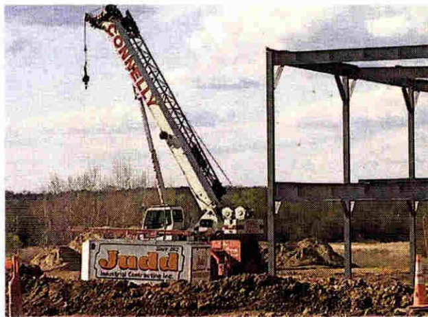
Construction is underway on the Northville Township side of Five Mile Road. ED WRIGHT/HOMETOWNLIFE.COM
