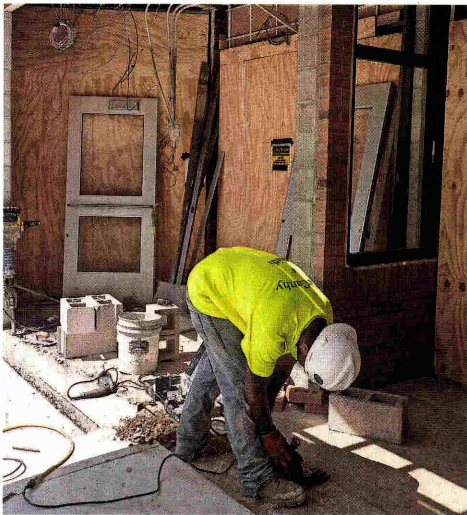
Ryan Lightfoot, of McCarthy & Smith Construction, works on the installation of the double set of doors at Beechview Elementary. BILL BRESLER | HOMETOWNLIFE.COM
