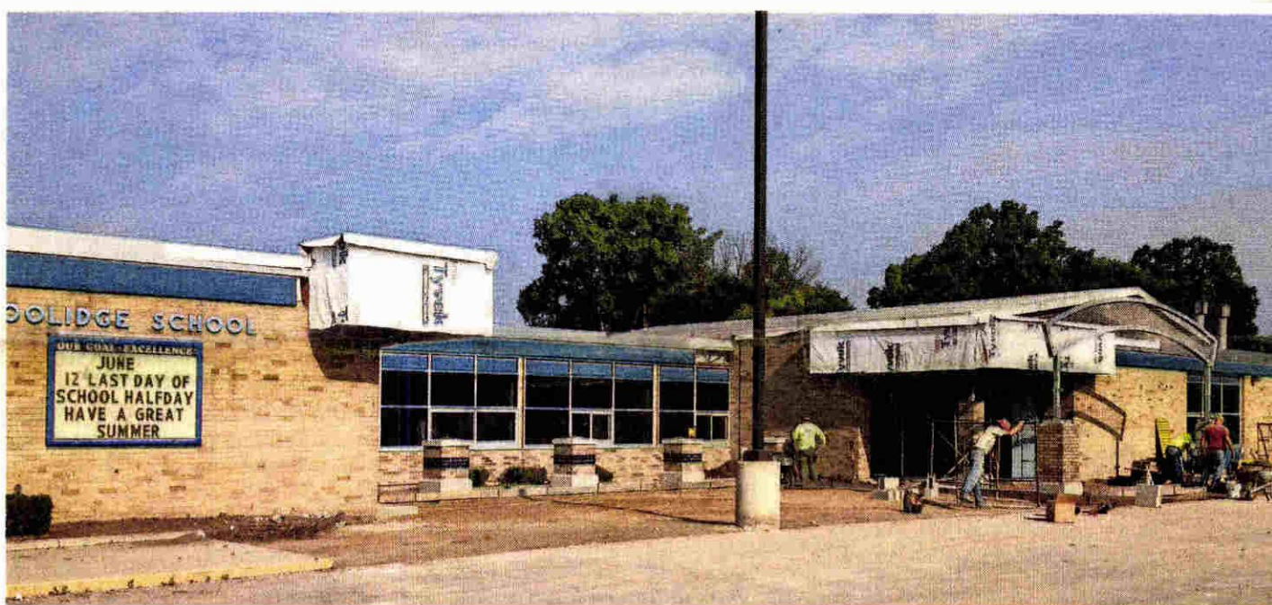
Workers continue their efforts improving the entrance at Livonia's Coolidge Elementary School. LIVONIA PUBLIC SCHOOLS
