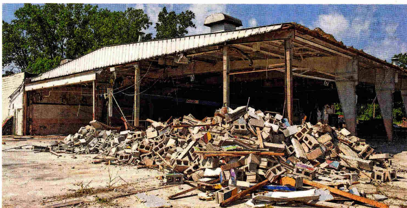
The former De-Sta-Co factory is partially demolished. Reconstruction of what is left will begin soon for the Village Arts Factory. BILL BRESLER | HOMETOWNLIFE.COM
