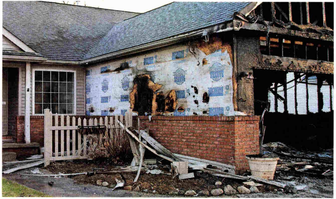
A fire Sunday damaged this garage at a house on Norfolk, west of Merriman. LIVONIA FIRE DEPARTMENT
