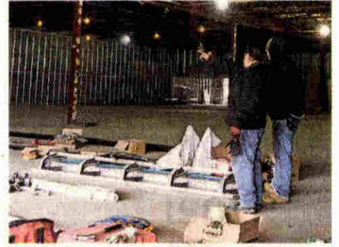
Planet Fitness is giving a makeover to the former Save-A-Lot site in Wayne. BILL BRESLER | HOMETOWNLIFE.COM
