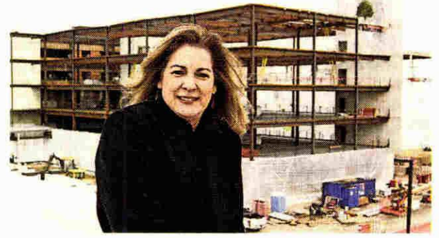
Beaumont President Connie O'Malley said the new emergency center should be open in December and the project completed by June 2019. BEAUMONT, FARMINGTON HILLS
