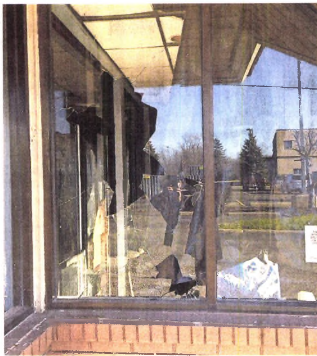
Vandals broke out a window of what is going to be a community center for New Hope Baptist Church in Wayne. NEW HOPE BAPTIST
