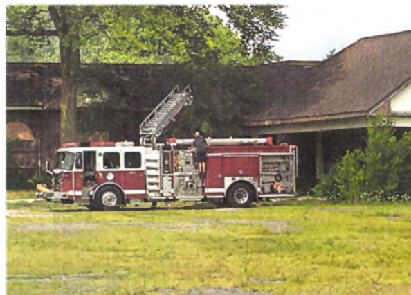
LEANNE ROGERS Westland firefighters found a fire at the former Hawthorne Valley from outside due to the poor condition of the building.
