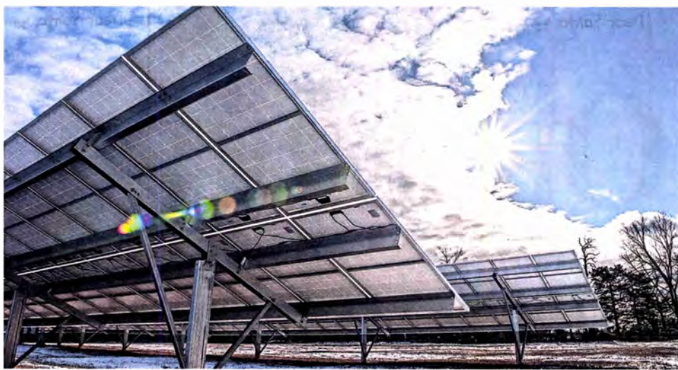
A large array of solar panels are mounted at the west end of the property, behind the Montessori School.
