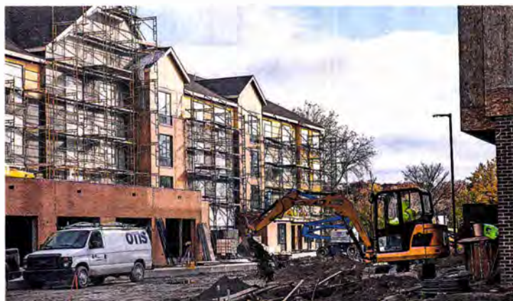
Bill Bresler | Staff Photographer New hotels are under construction just west of I-275, changing the face of the Ford Road corridor.
