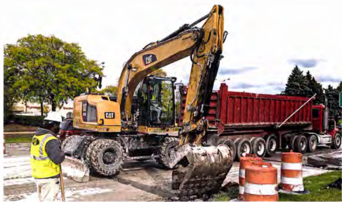
BILL BRESLER | STAFF PHOTOGRAPHER Road construction crews remove old roadway and curbs before replacing the road surface.
