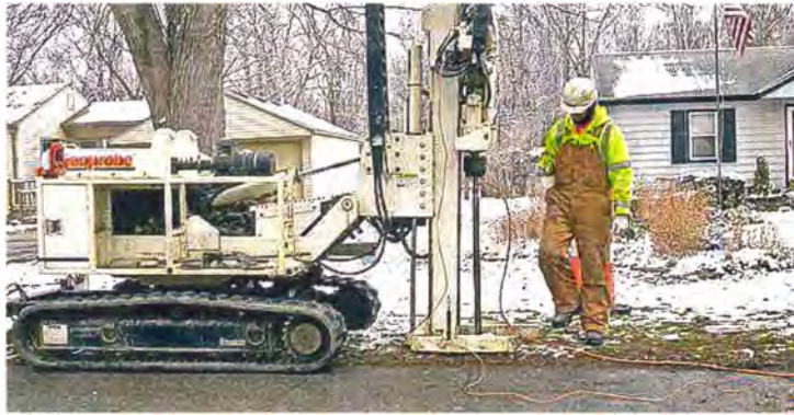
A worker drills in the Alden Village subdivision earlier this year. Ford says it has identified the extent of groundwater contamination in the area and will work to monitor it in the long run.
