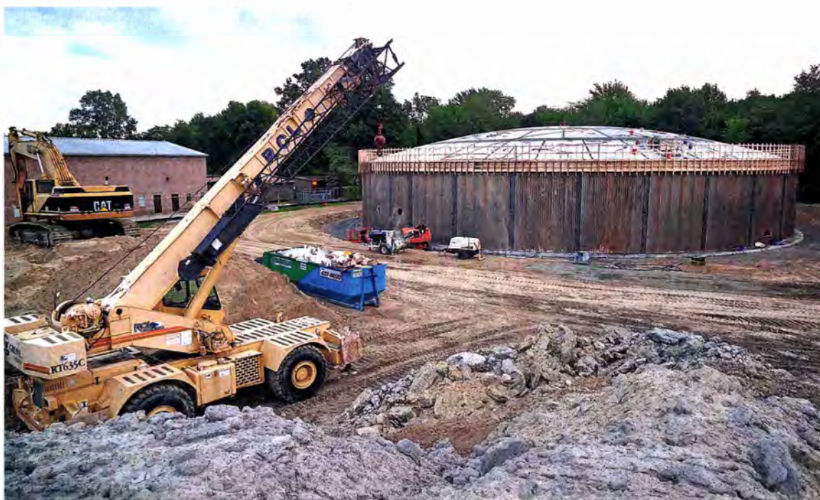
The storage tank will fill at non-peak usage hours and allow Canton to release water during peak hours, placing less strain on the system.
