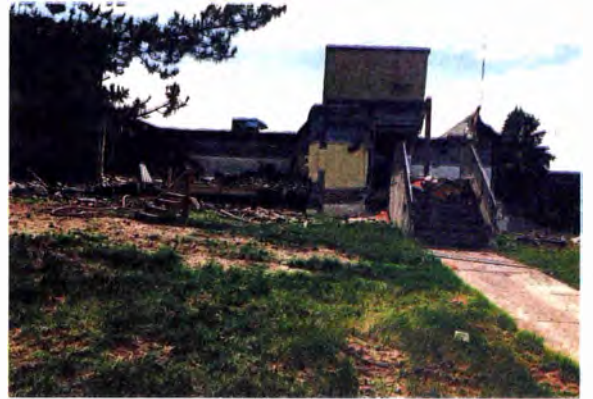
The east side of the closed Bailey Recreation Center as demolition gets underway.
