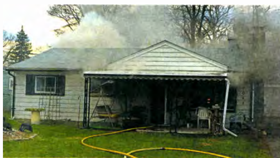
WAYNE-WESTLAND FIRE DEPARTMENT The fire at this home in the 33000 block caused extensive smoke and water damage.
