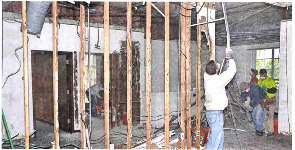
Crews work on the factory on the 14-acre site at Ridge and Cherry Hill roads.
