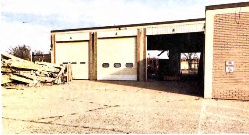
Long a fixture on Ford Road, Westland's old fire station one is being demolished.
