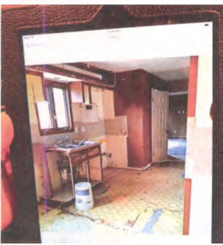
JOHN HEIDER | STAFF PHOTOGRAPHER Sharon Drochak displays a photo on her tablet computer that shows how her kitchen looked at the beginning of the renovation.
