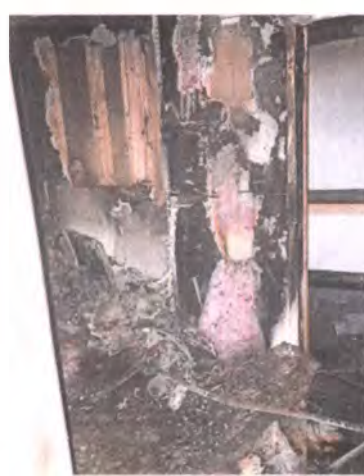
WAYNE-WESTLAND FIRE DEPARTMENT A fire that killed a Westhaven Manor resident started in the closet of the apartment.
