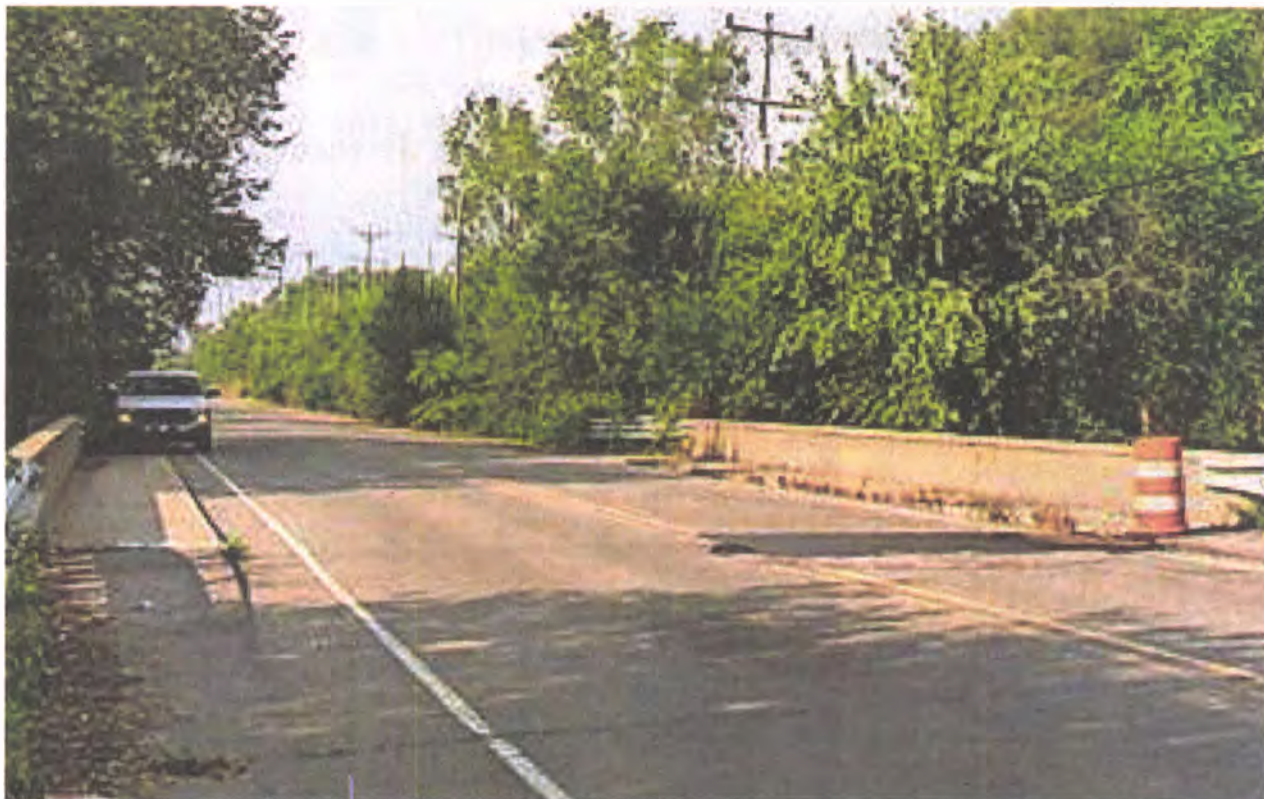
The storm-damaged bridge on Henry Ruff just north Michigan Avenue will be repaired beginning next month. The bridge will be closed during the construction.
