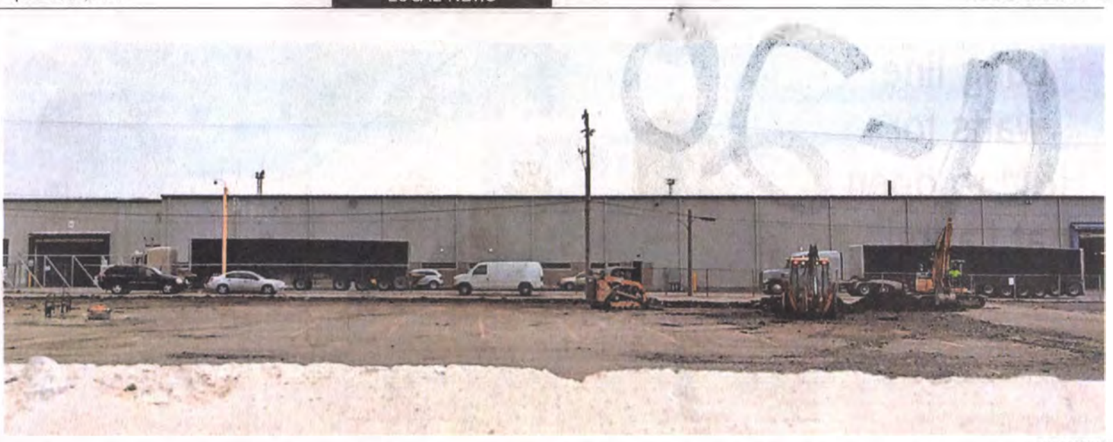
Heavy equipment has started removing a portion of the Wayne Commons parking lot that has been walled off from the remainder of the strip mall.
