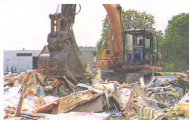
A pile of rubble is all that is left of the vacant Westland Economic Development building.
