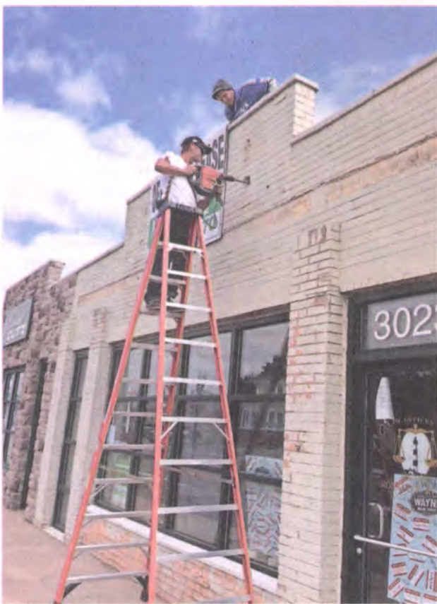
Jimmy Slees (left) and Ken McCarthy of C.F. Electric work on lowering exterior lighting on the front of Paul Visingardi's building on Wayne Road.
