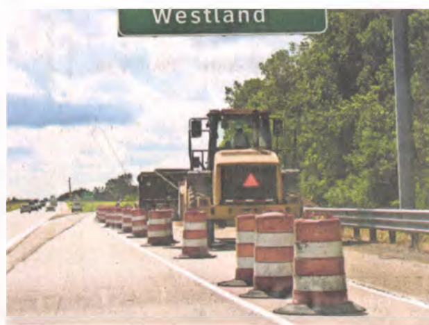
Shoulder work is occurring along the southbound I-275 exit to Ford Road.
