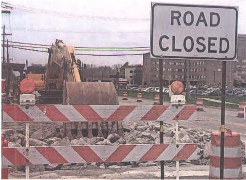
FILE PHOTO Current sewer work being performed on Levan near Five Mile. The road between Schoolcraft and Five Mile will see some closures this summer as it's resurfaced beginning in June.
