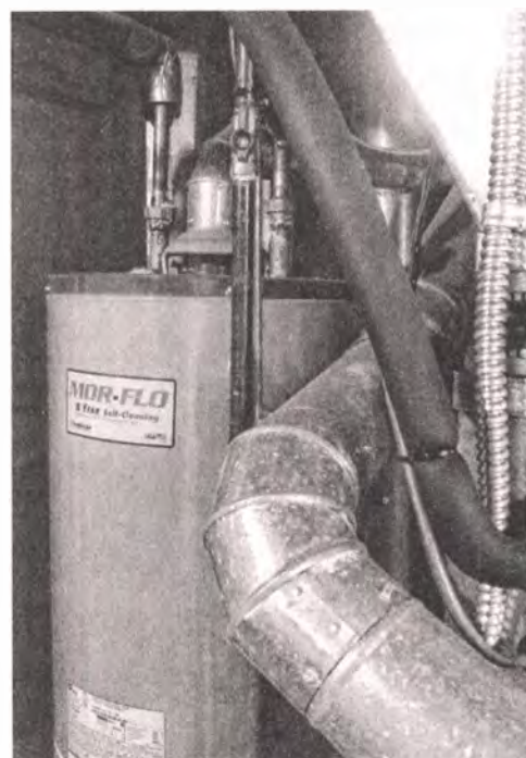
Newer, bigger hot water heaters may not fit into existing cramped basement spaces. SUBMITTED
