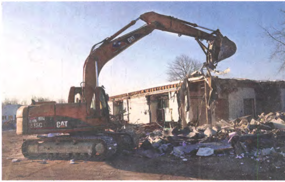
Demolition began in December on Nankin Mills School. The school board hired a firm Monday to market the seven-acre property, as well as the 10-acre site of the former Washington School, which was torn down in 2014.
