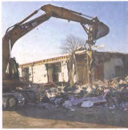
BILL BRESLER | STAFF PHOTOGRAPHER Demolition began on Nankin Mills School in December. The site is one of five properties the Livonia school board is considering selling over the next couple of years.
