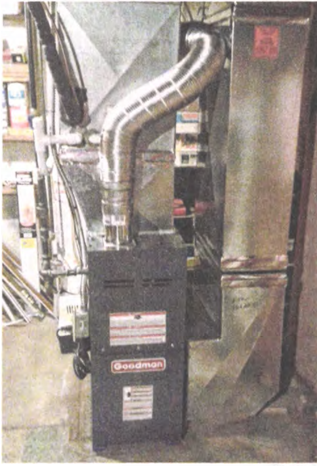
The finished product is a more efficient furnace — all free of charge, thanks to SEMIACCA members.
