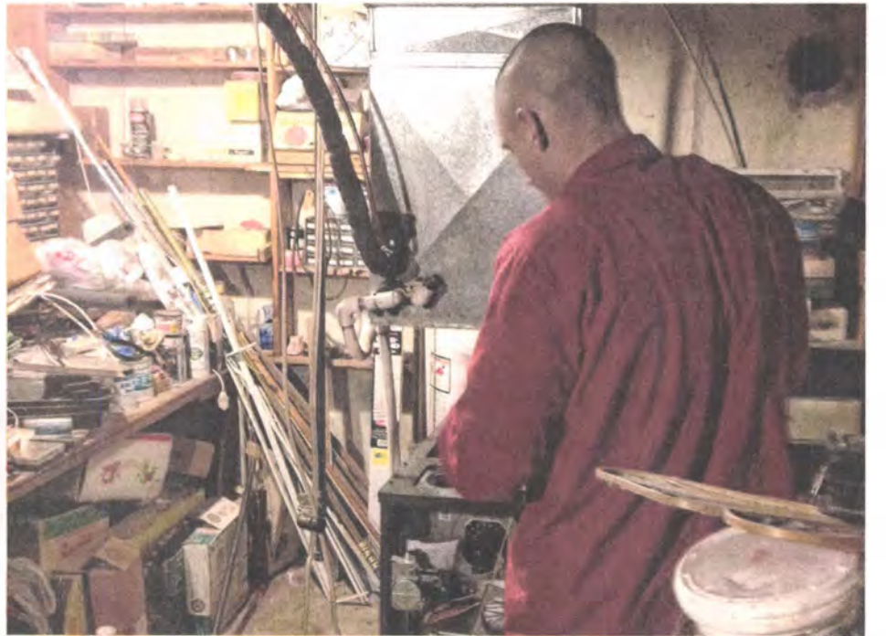
Dan Palko sizes up the work needed to properly install the new furnace.
