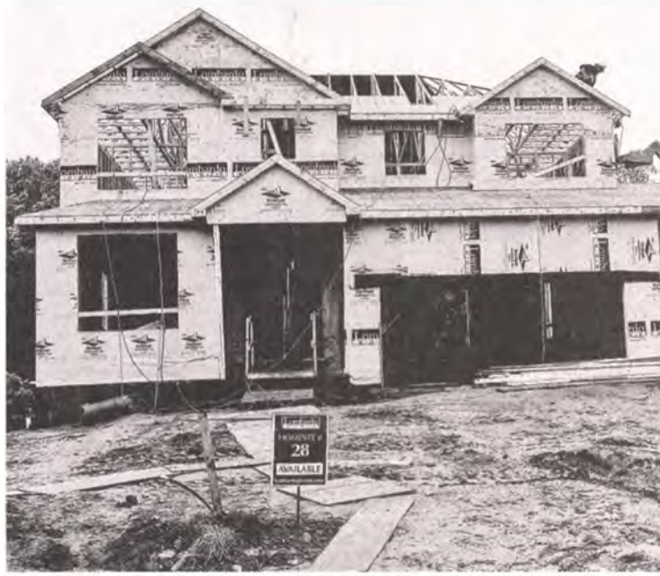
Homes are and have been under construction throughout Lyon Township, like this one.
