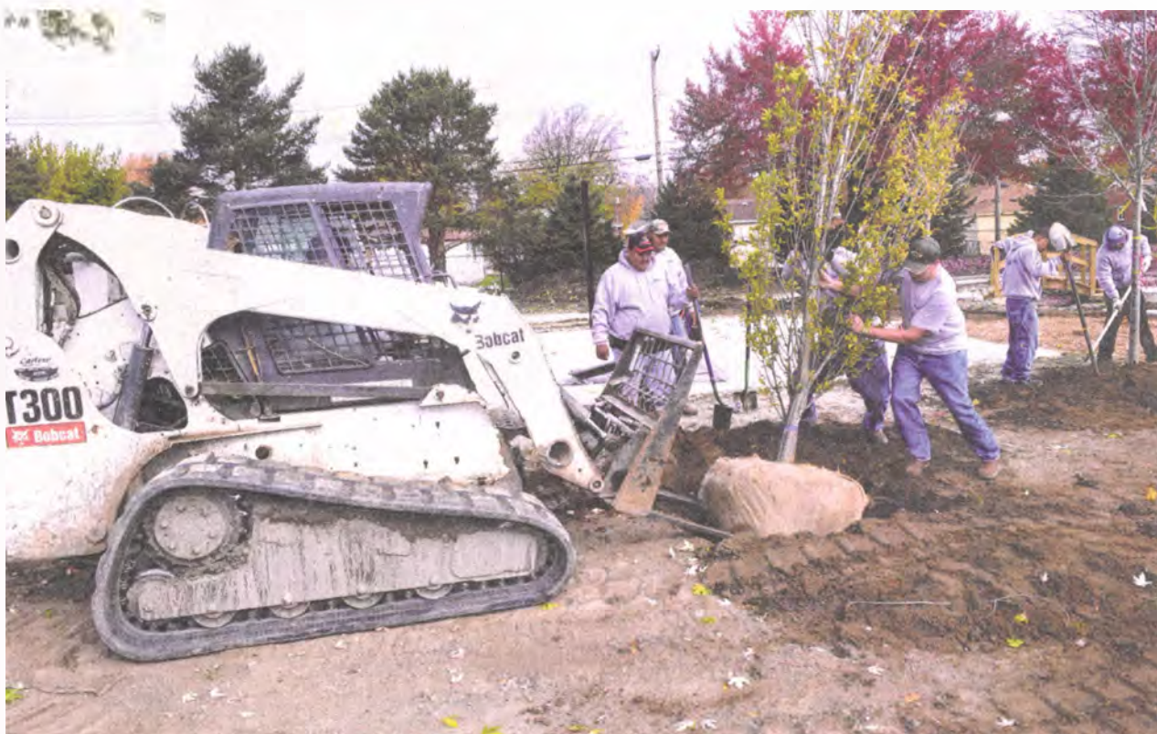
Dozens of landscapers and other volunteers helped to finish the project at the First Step shelter in Wayne.
