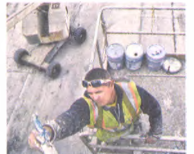
Bill Bresler | Staff Photographer Domenic Rolak of G and M Painting paints the Berwyn Street bridge in Redford.
