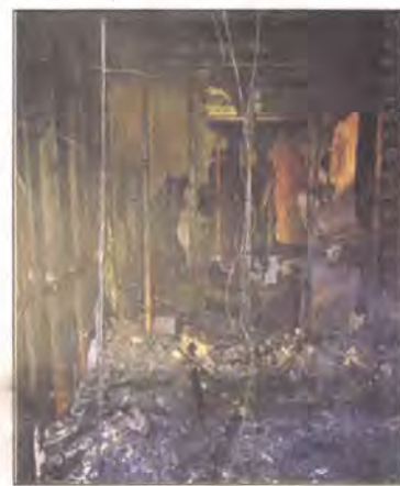
This garage apartment was destroyed by fire early Tuesday.
