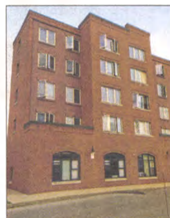
Newberry Square tenants have opened their windows to get air into their apartments.
