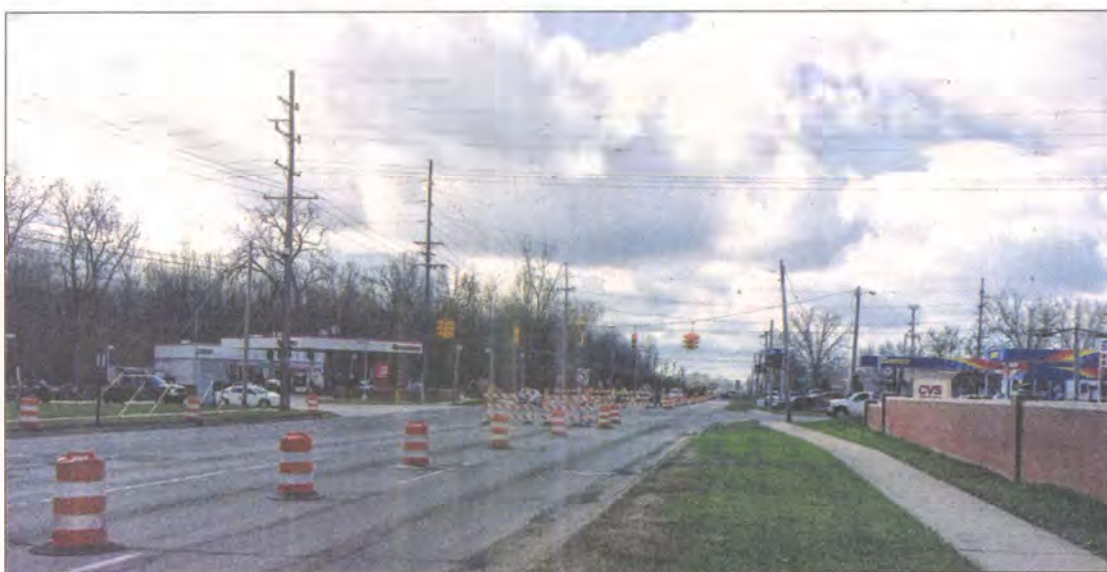
Orange barrels sat along Newburgh at Cherry Hill on Thursday, when work began on improving the intersection and traffic signal.
