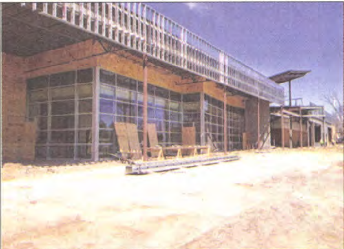
As work on the new Westland City Hall progresses, little is left of its previous life as a Circuit City store.
