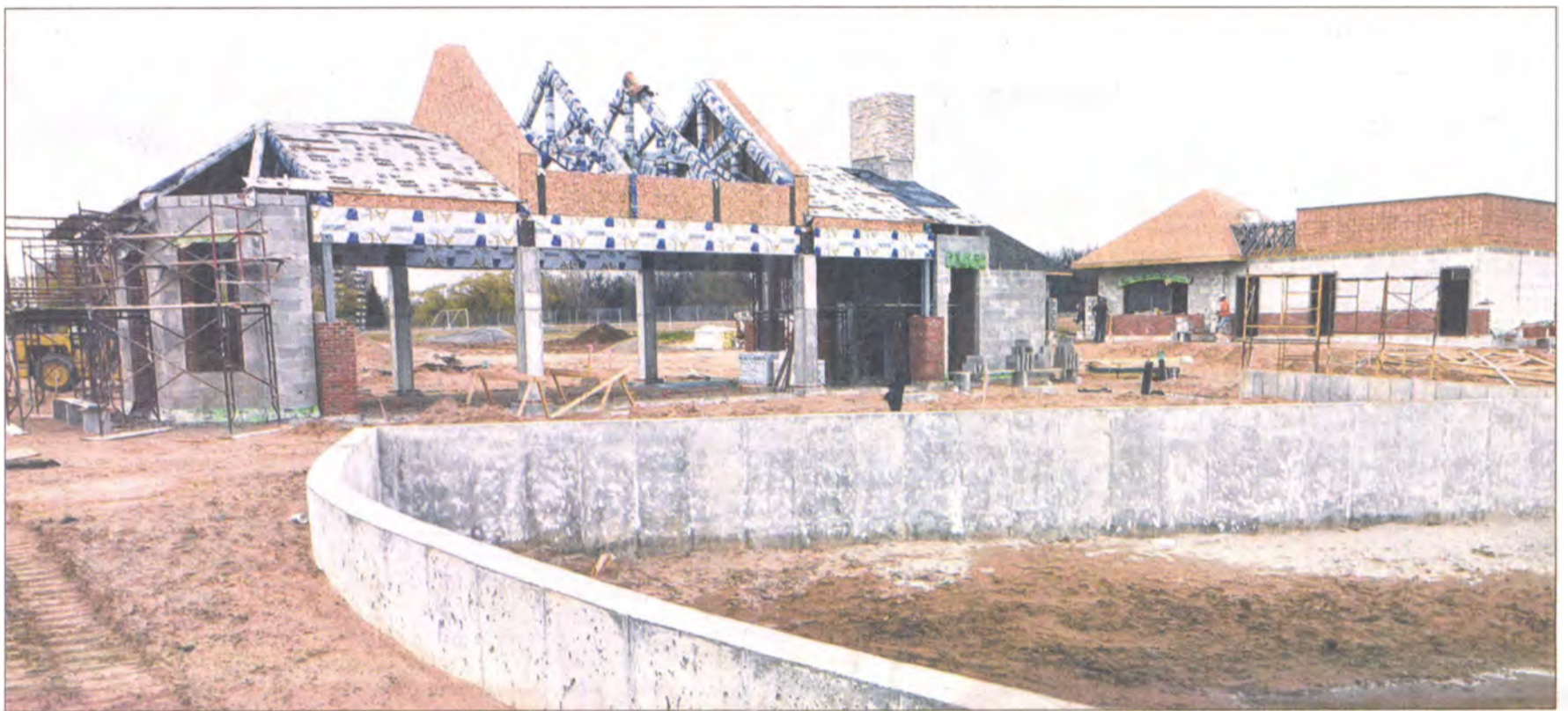
With the break in winter weather, construction on the Westland Farmers Market Pavilion continues. PHOTOS BY BILL BRESLER | STAFF PHOTOGRAPHER
