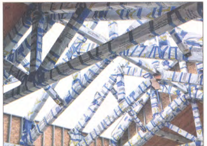
Still open to the sky, construction continues on the Farmers Market Pavilion in Tattam Park.
