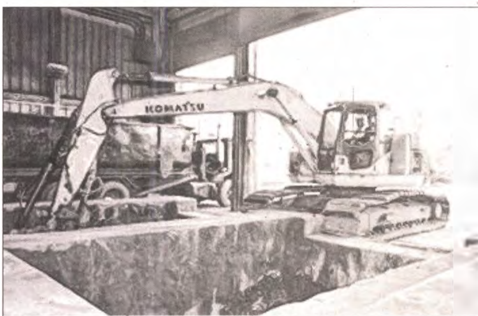
EQ offers a delisting treatment process which converts hazardous inorganic wastes into non-hazardous, delisted residuals.
